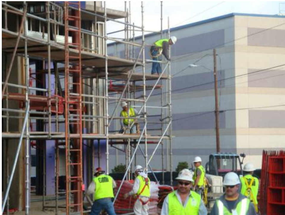
Safety trained GMi scaffold crew go to work on scaffold erection for 8 story multi-family job.
